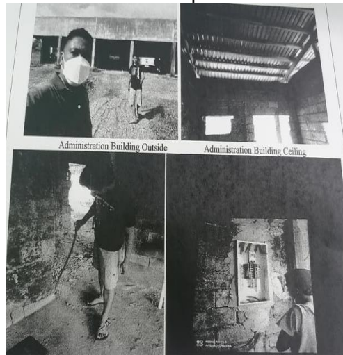
Multi-Purpose Evacuation Center, Water Refilling Station, Administration Building (PH.2) & Drilling/Installation of Water System w/Submersible Pump.
