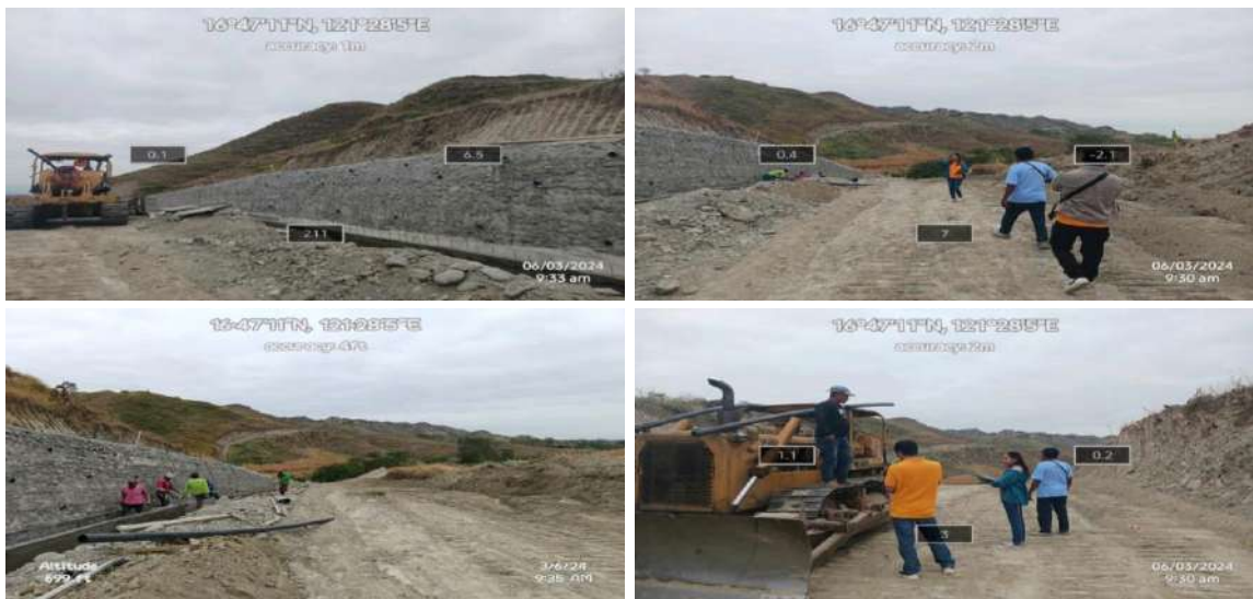
Area 1: The on-going construction of access road leading to the Rolling Hills, within Barangay Planas-San Miuuel-Aaualdo. Ramon, Isabela.
