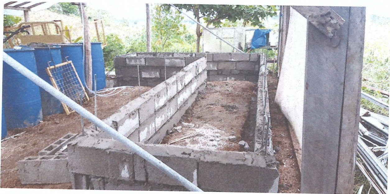
Construction of vermi bed for the production of organic fertilizer for use in the production of Assorted vegetable seedlings and organic vegetable garden.
